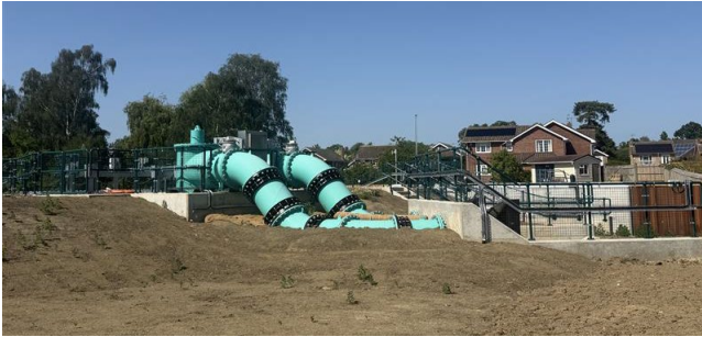
Above: The new Hildenborough Pump Station
