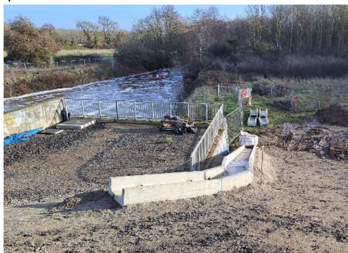
The new eel pass structure being constructed next to the Leigh control structure
